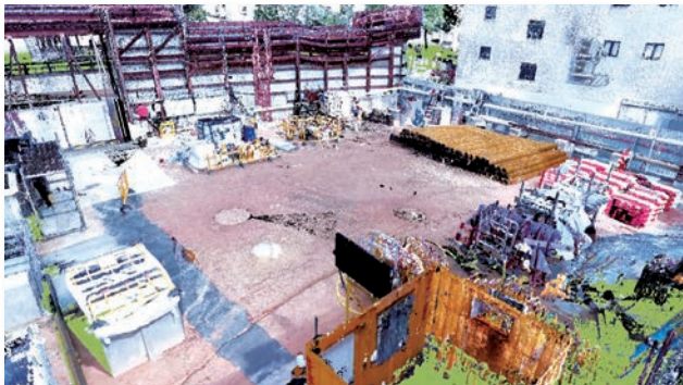
Point cloud technology can show site environment at real-time via laser scanner
