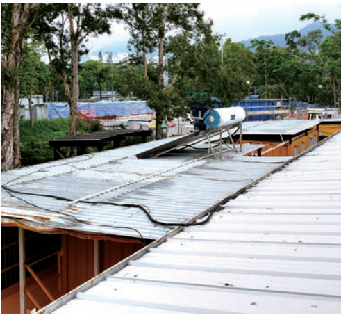
Renewable energy water heater system
