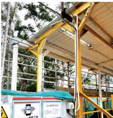
Rainwater cooling system
